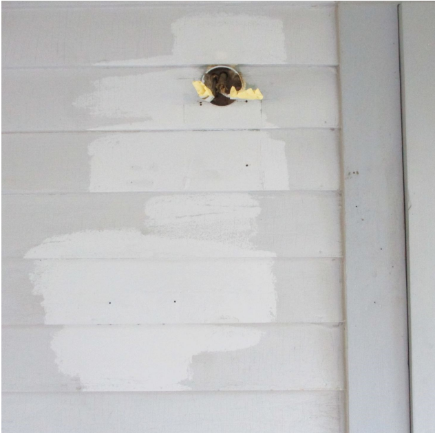
Front porch light temporarily disabled. Back porch light, out of commission.
